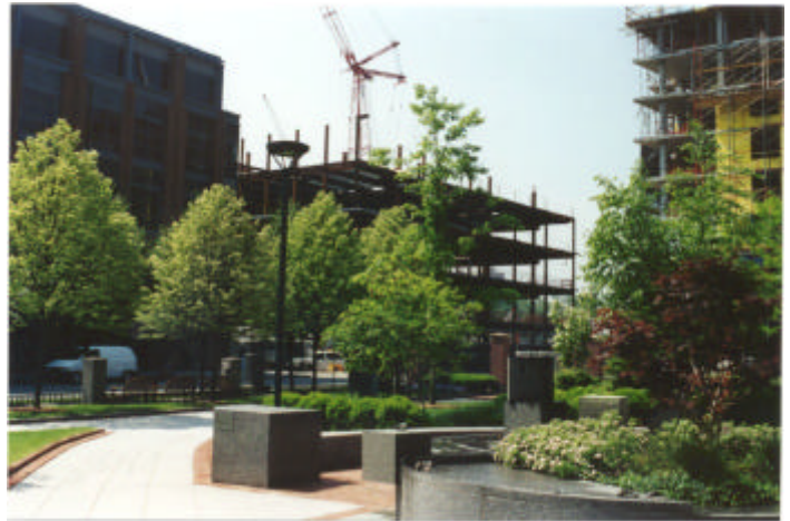
Rising next to the current HQ at 64 Sidney St. in Cambridge, 88 Sidney Street is an 145,275 sq.ft. build-to-suit office/lab project for Alkermes, Inc.
