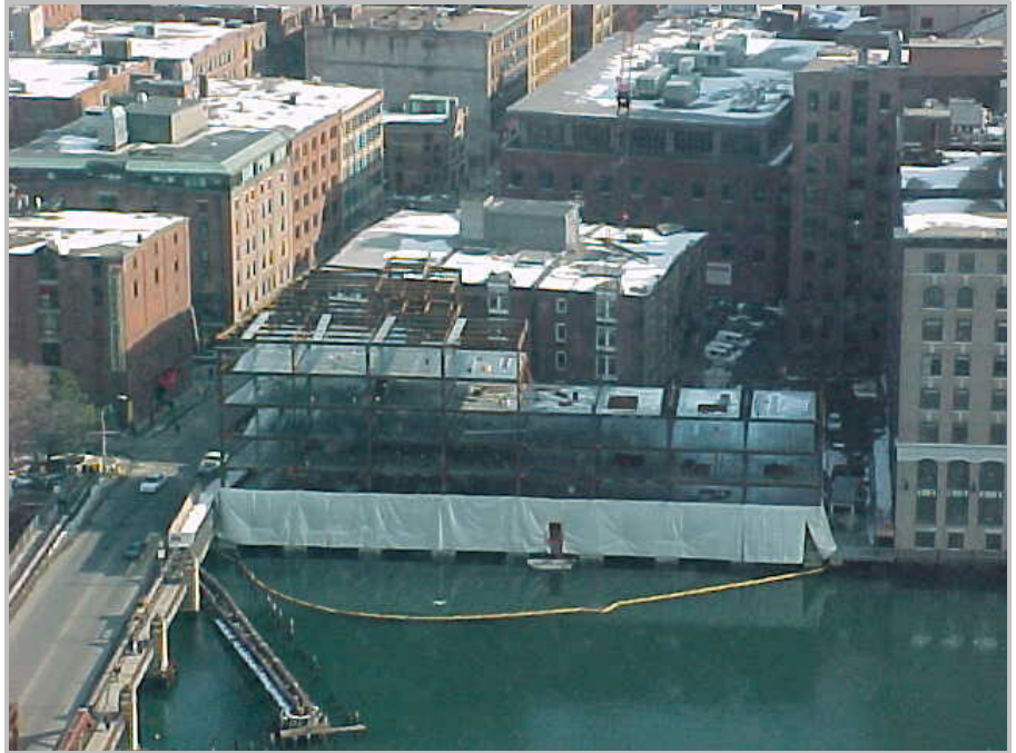
303 Congress Street (shown under construction on the east bank of Fort Point Channel) will add 65,728 square feet of Class A office and retail space to the Boston Central Business District in 2001.
